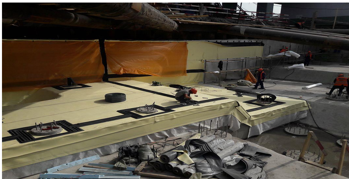
Figure 2. Installation of a membrane for vertical waterproofing of the foundation, work is carried out in the pit along the wall in the ground system, scaffolding is used
